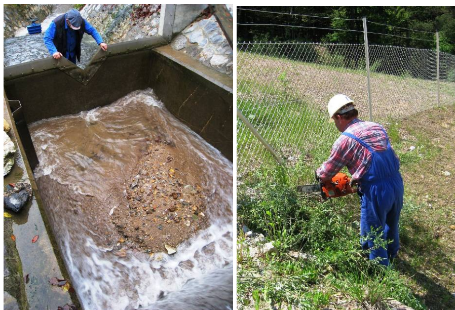
Figure 21: Cleaning the deposits of the measuring point after a rainfall (left) and removing the bushes along the protective fence at the Boršt disposal site (right)
